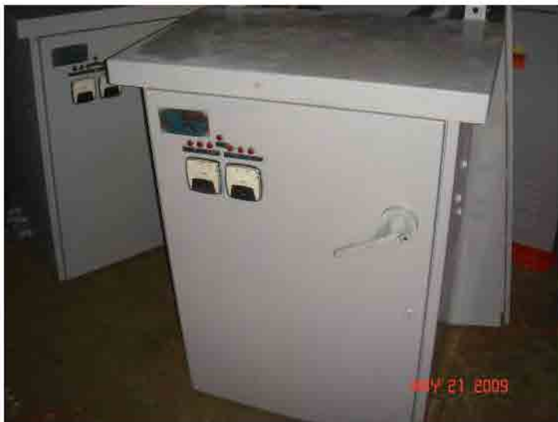
1(c-1) & 2(c-1) Walker transformer & controller
