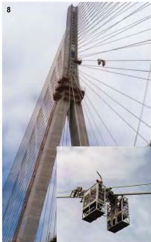
8 - Freely suspended cradle for inspection and maintenance of guy ropes on suspension bridge (Normandy Bridge). Powered TIRAK hoists and power pack mounted on the cradle.
