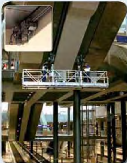
Double ACS rail with special platform, Main Station Berlin (D)
