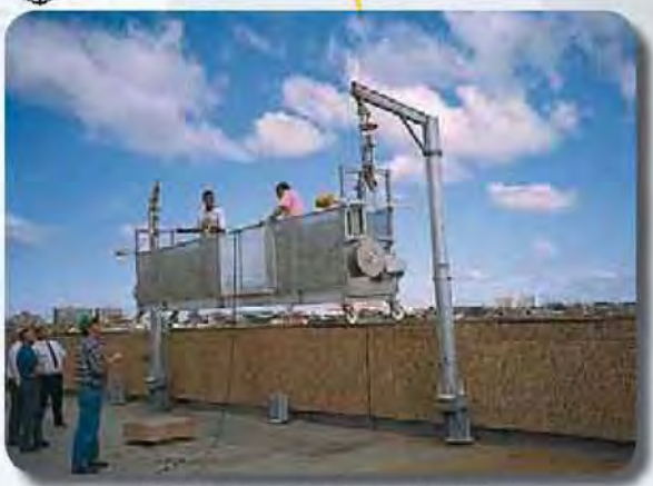
Suspended powered platform on 2 Davits (ZA)
