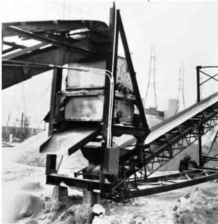
Single Stage DF Separator removing ferrous contamination from slag for use in cement block manufacture.
