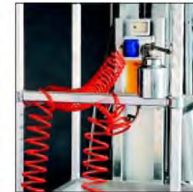
compressed air or water connector on platform
