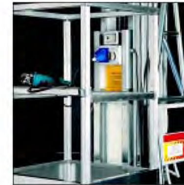
220V single phase socket with switch for power tools.
